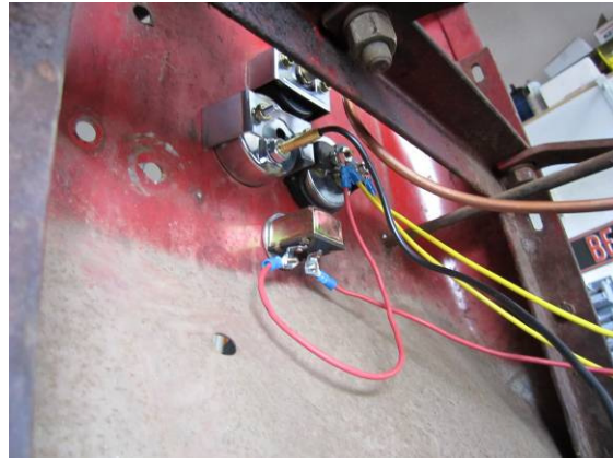
Wiring behind gauge panel
